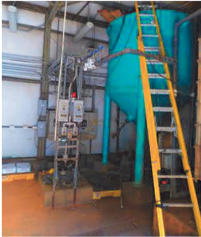
Interior of the BV groundwater treatment system building (the system has been decommissioned)
