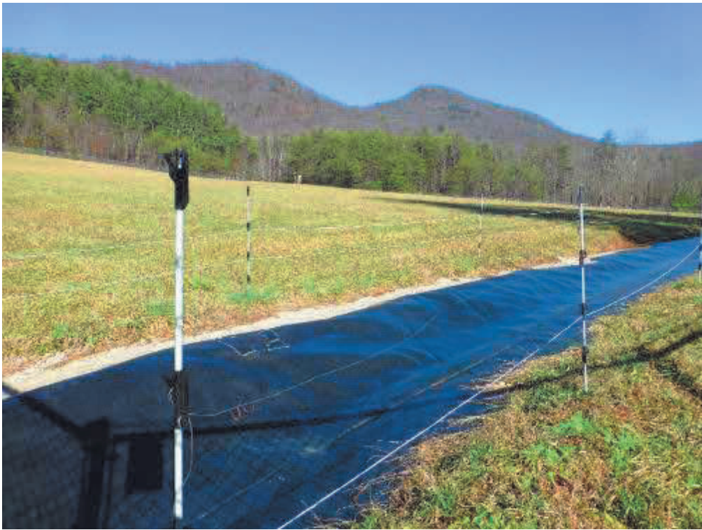
APA with new stormwater diversion swale
