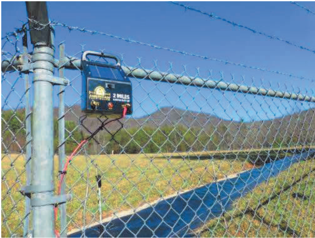
Solar-powered electric fence installed around APA stormwater diversion culvert to deter wildlife
