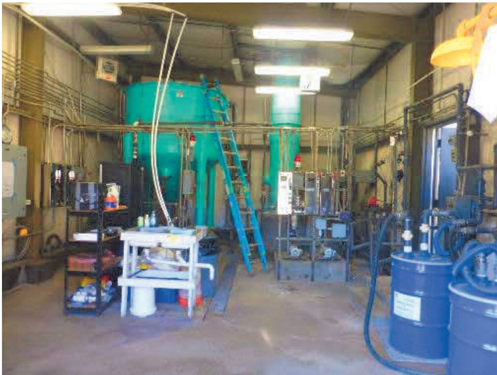
Interior of the FV groundwater treatment system building
